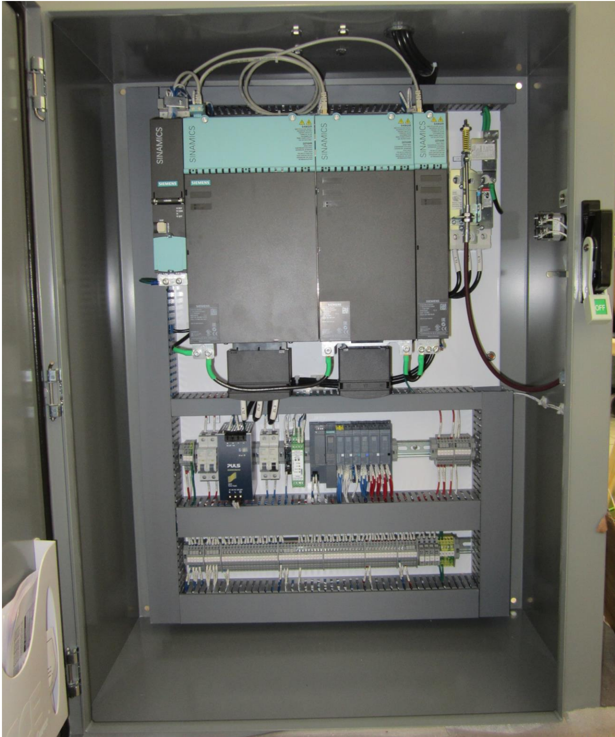
Wire drawing control panel shows the heart of this solution, the SINAMICS S120 Drive.
